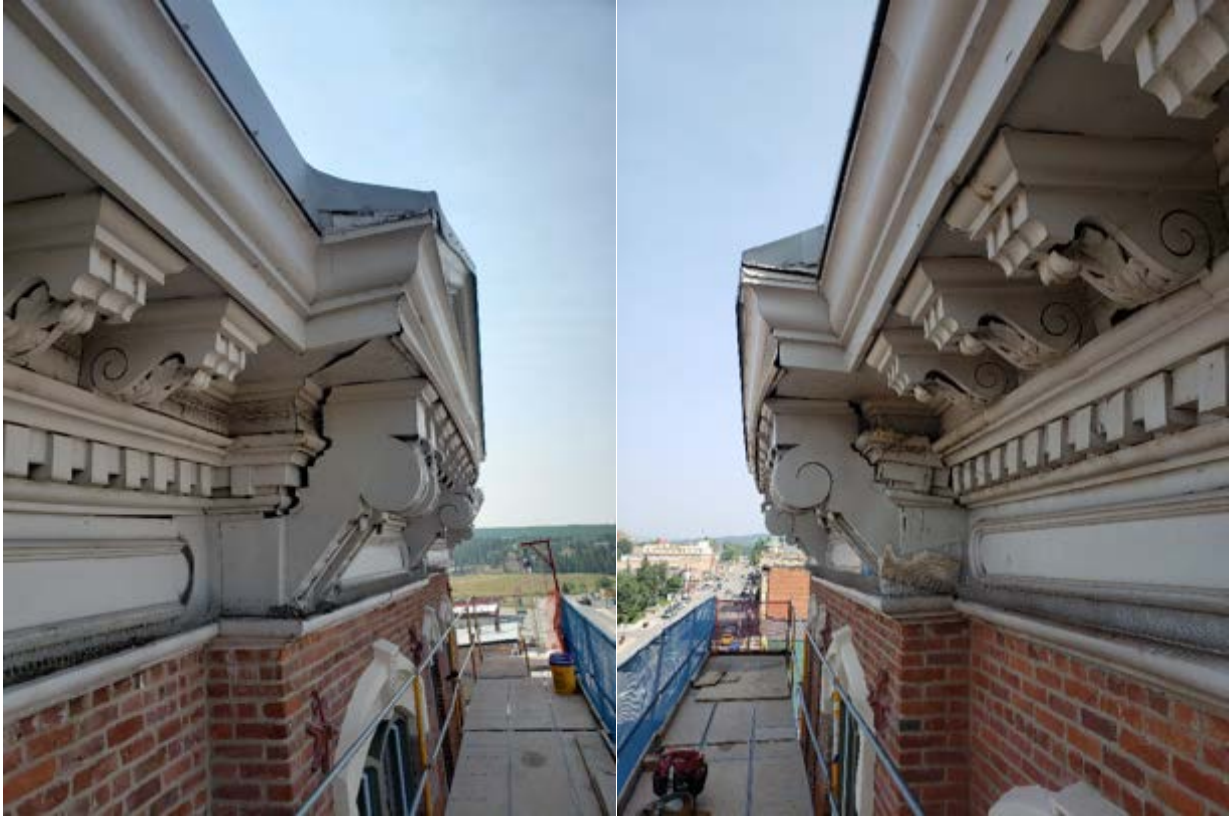
Cornice bulging and pitching forward, particularly at the central bump out.
