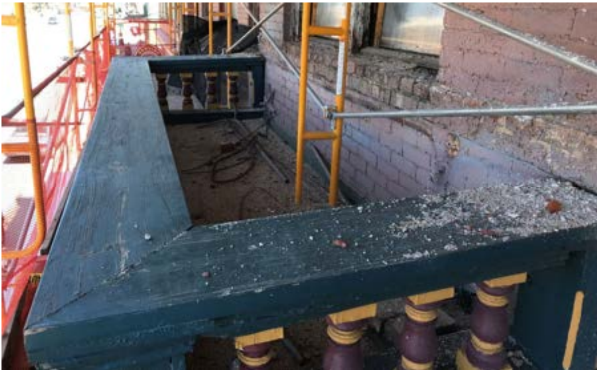
Image 16 – Balcony – Looking north. The scaffolding allowed a close-up view of the balcony during the rehabilitation of the masonry and windows in 2021. The original wood balustrade cap with separate newel post caps was replaced sometime after images 14 & 15 were taken. The balustrade cap will be returned to its original design.
