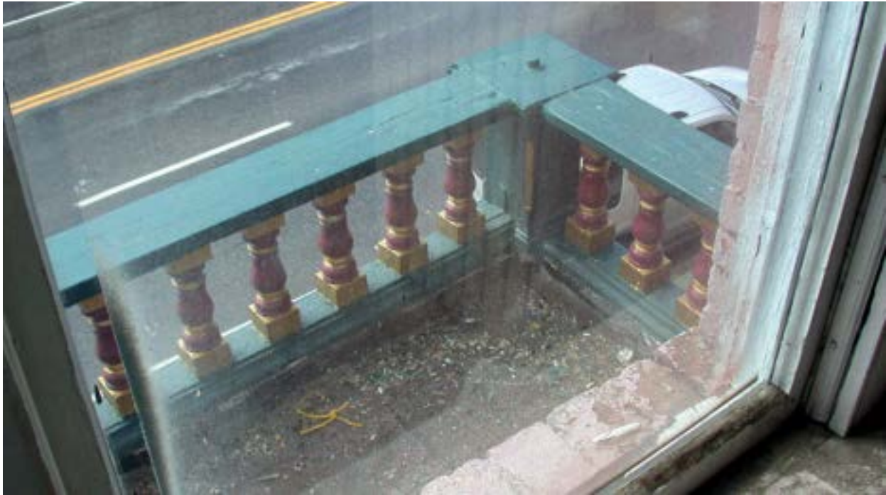
Image 15 – Balcony – North end. Following the removal of the existing modified bituminous sheet roofing, the condition of the underlying wood flooring and balcony framing will be reviewed and replaced where rotted. New single ply membrane roofing will be installed following repairs. The floor will be sloped to an original scupper, located on the east side of the balcony floor.
