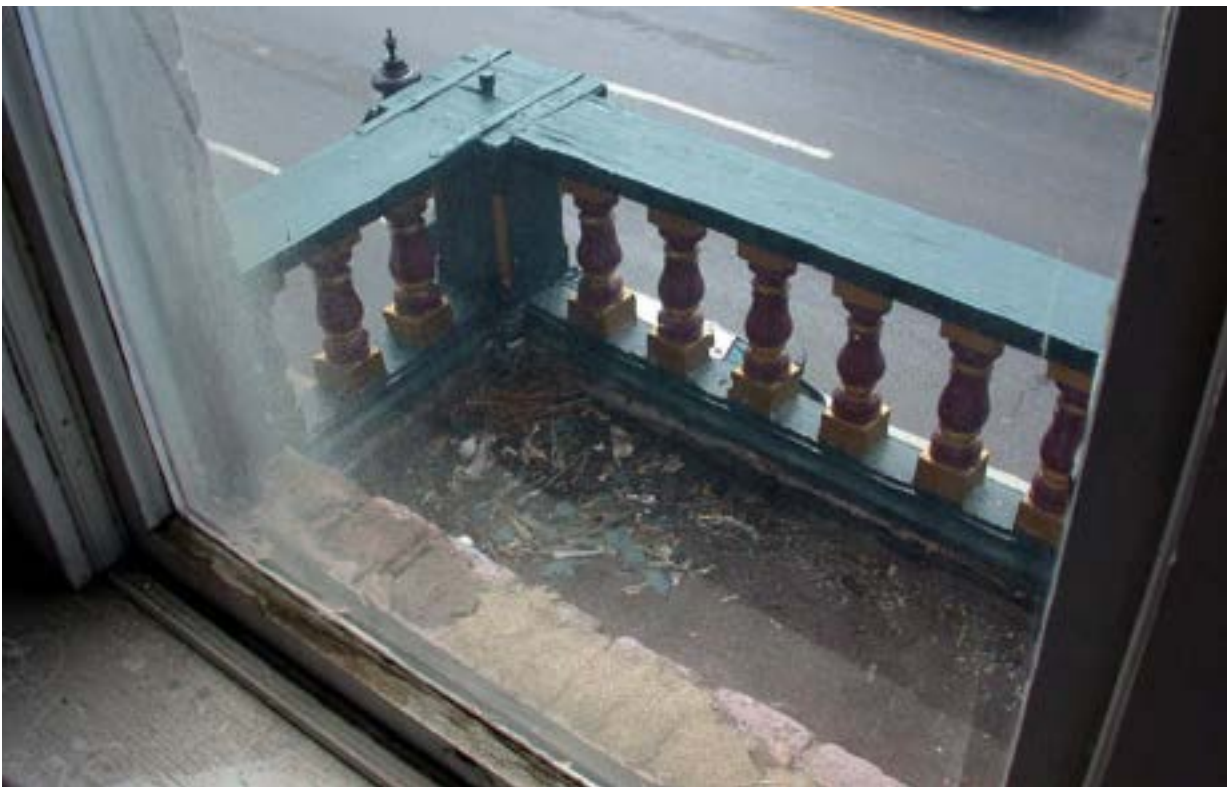
Image 14 – Balcony – South end. This view from a second floor window reveals the condition of the balcony. Loose paint chips have collected on the balcony floor. The wood at the balustrade's bottom rail is likely in poor condition due to moisture infiltration. Deteriorated wood will be replaced in-kind. Balcony components will be checked for secure attachment.
