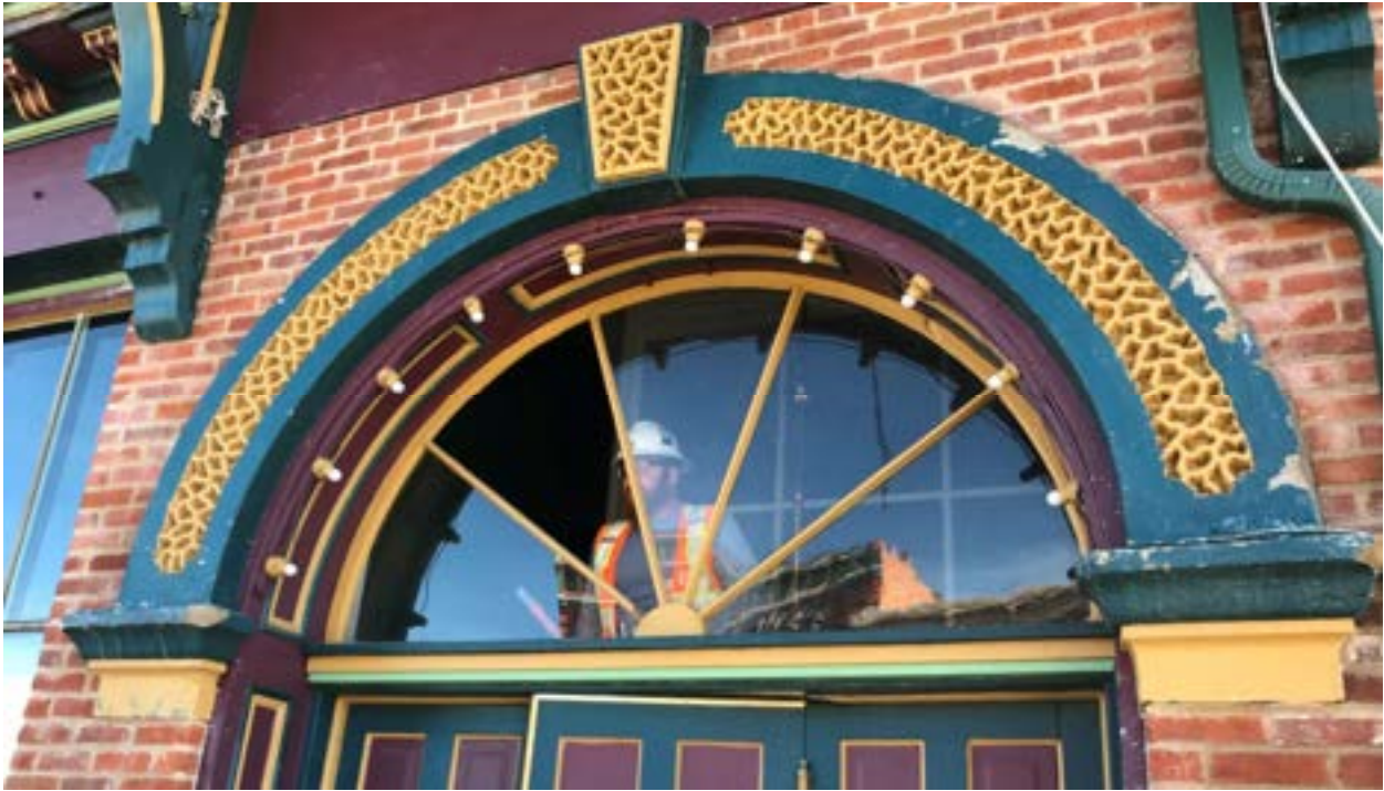
Image 8 – Central Main Entry with semi-circular transom above. The decorative lighting around the fanlight window poses a safety hazard due to the condition of the exposed wiring. Loose and peeling paint will be carefully removed from the ornamental plaster arch and keystone and then repainted as part of the historic paint scheme for the building.
