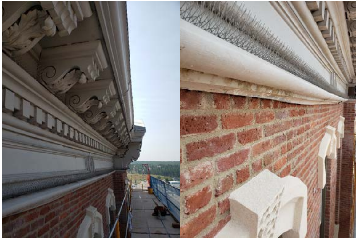
Waviness of the cornice bottom plate and consequent irregularity of top visible row of bricks
