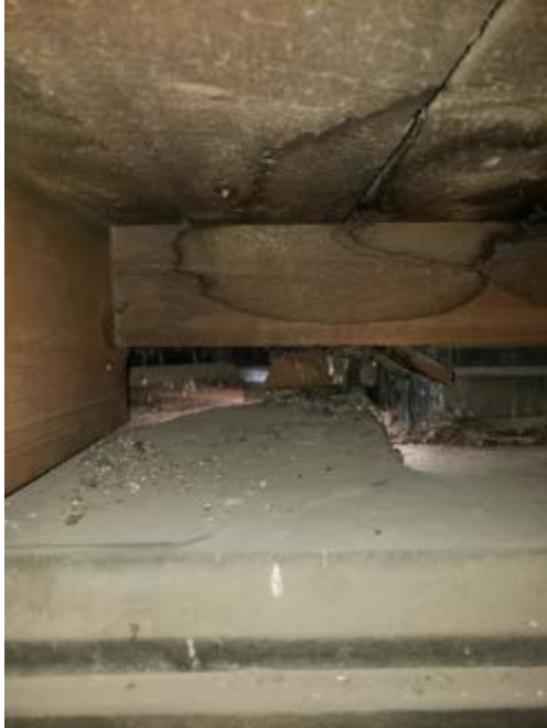
Water stains on decking and roof members
