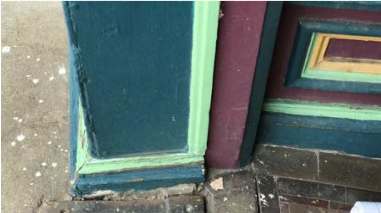
Image 13 – South Storefront – Close-up of column base. The poor condition of the wood trim can be seen here. Paint is missing in many locations while in other locations, it is built up, requiring its removal. Wood trim beyond repair will be replaced in-kind, matching historic profiles.
