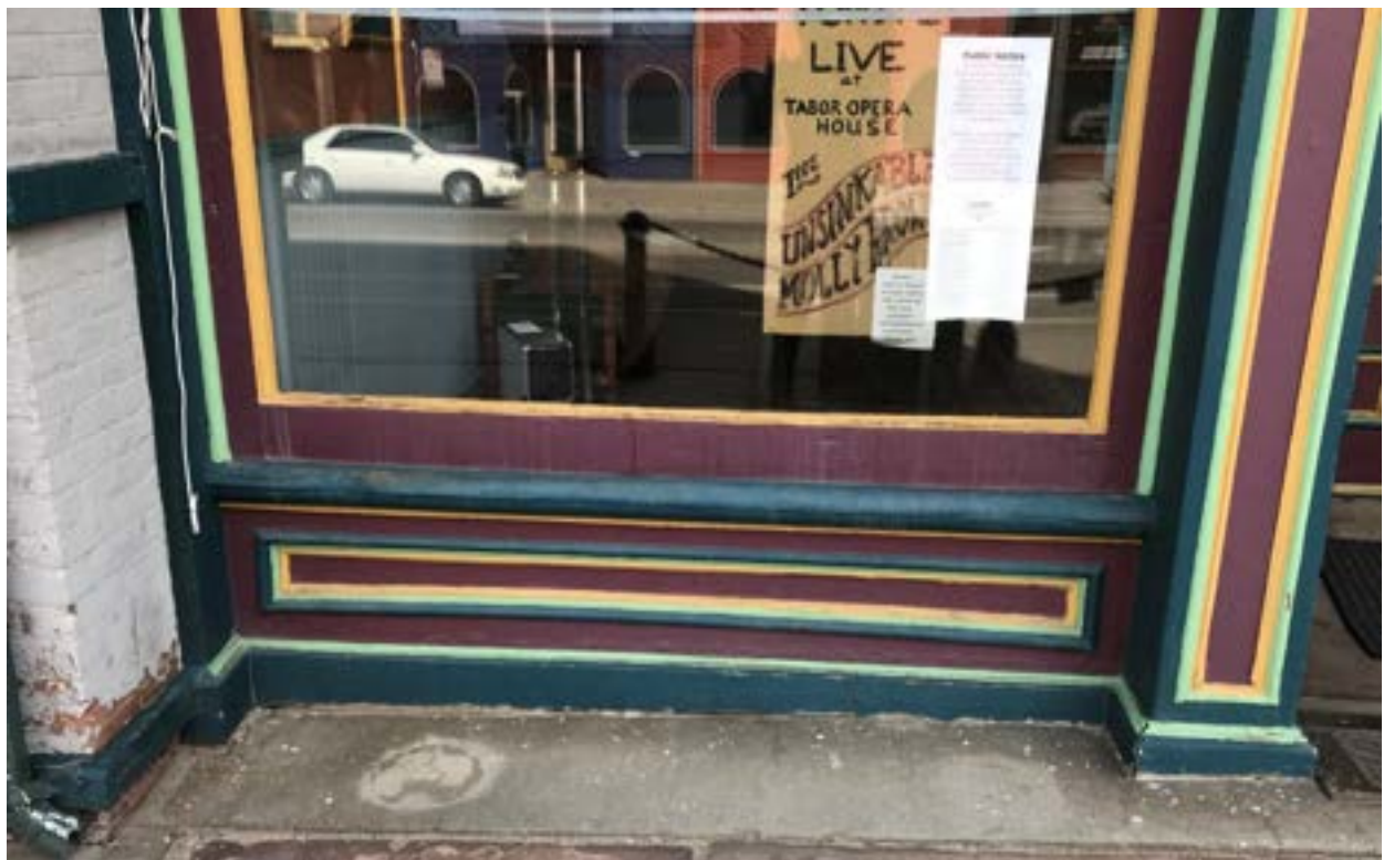
Image 9 - South Storefront – Partial view of north side. Paint is missing from the wood trim. Wood close to grade is especially in poor condition due to moisture infiltration. Trim will be replaced in-kind, matching historic profiles.
