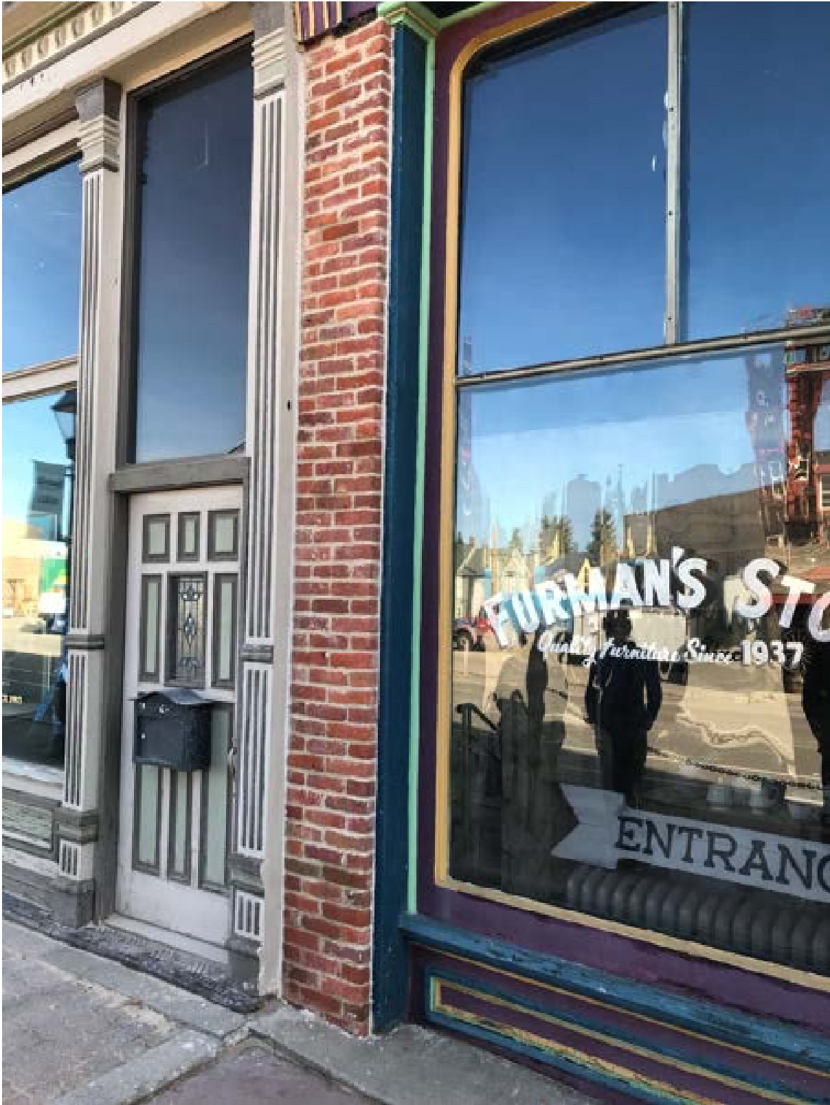
Image 6 - North Storefront – View of north end. The alligatored and peeling paint will be removed from the wood trim. Where the wood is close to grade, a paintable water-repellant wood preservative will be applied. Where a sealant or caulk is required to fill open cracks or joints in the woodwork, a high quality exterior primer will be applied. Storefront windows will be checked for secure attachment to the window frames; wood stops will be replaced as required.
