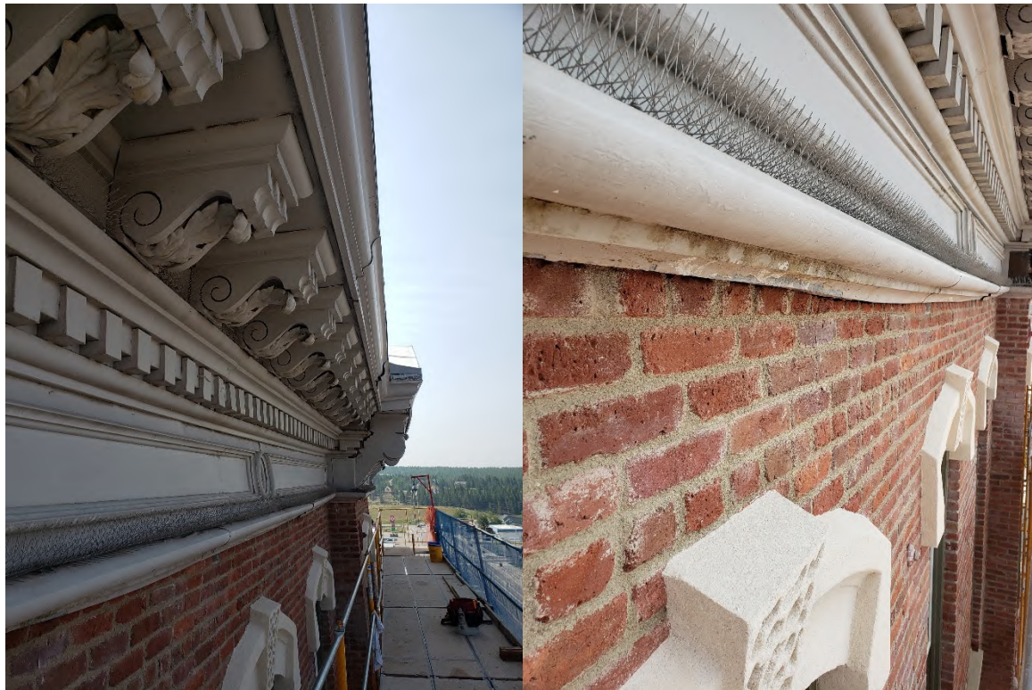
Waviness of the cornice bottom plate and consequent irregularity of top visible row of bricks
