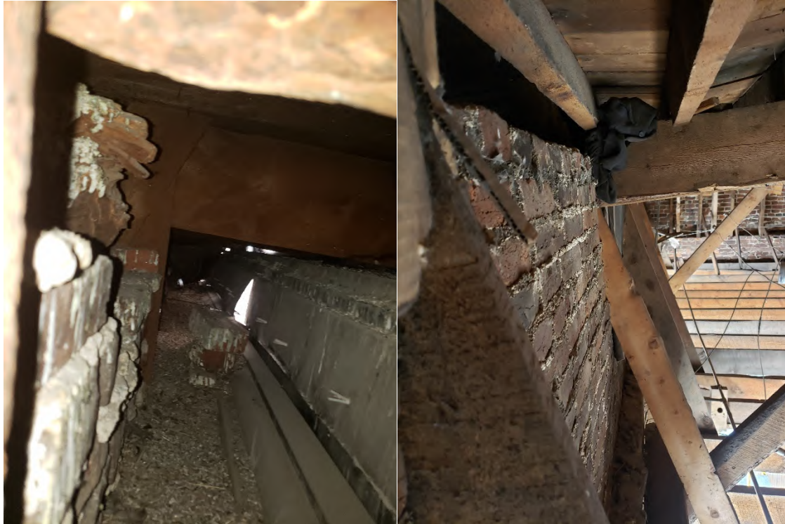
More upper cornice framing details, including diagonal attachment to ceiling joists below
