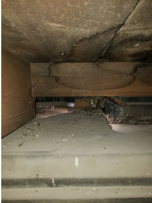
Water stains on decking and roof members
