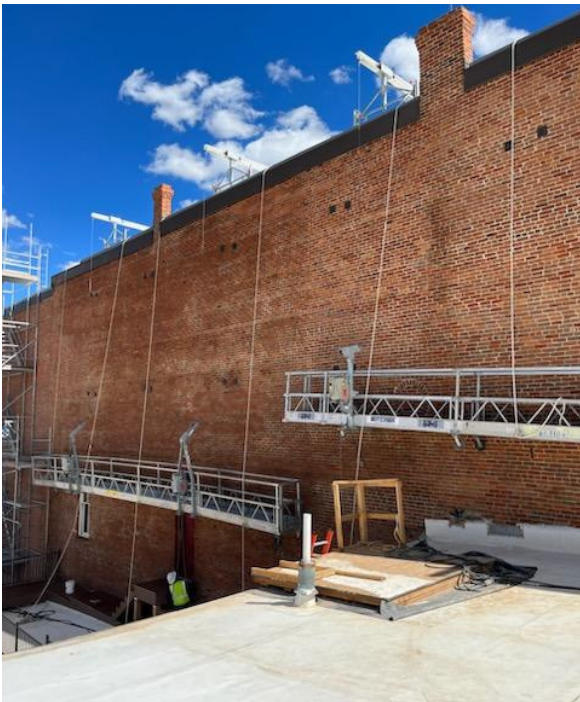
The scaffolding on the Tabor's north wall-used a swing stage system for 2023 construction
